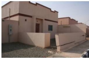
Picture (5) the cracks and collapse of one of the housing units
