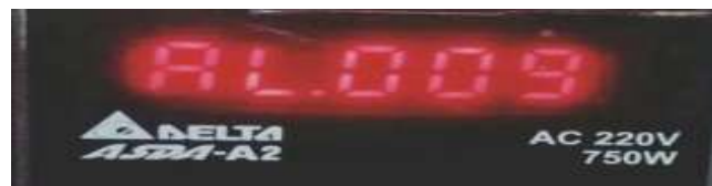
Figure1: Alarm display panel.
