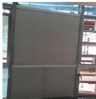
Fig.7: Installing Jensen board on the aluminum units of the skin not on its units Source:
