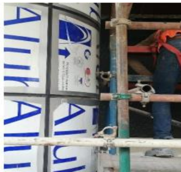
Fig. 12: scratches on building skin column cladding units Source: Researchers
