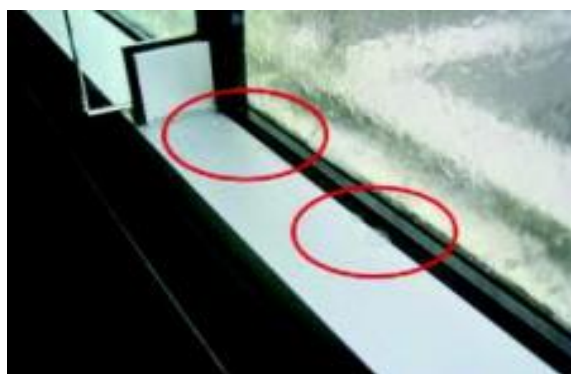
Fig. 4 (A): (Installation issues)Water ingress observed during laboratory static water penetration resistance testing. Source: [1]
