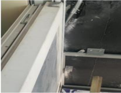
Fig.8: Installing Jebesen board on the aluminum units of the skinned on its units Source: Researcher
