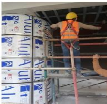
Fig. 11: scratches on building skin column cladding units Source: Researchers
