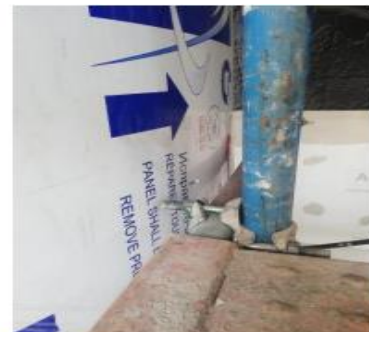
Fig.13: scratches on building skin column cladding units Source: Researchers
