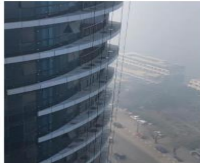
Fig.9: Water spots on building's cladding Source: Researcher
