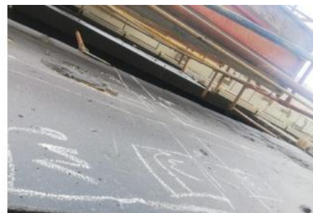
Fig.16: m Extra part in concrete must be removed Source: Researcher
