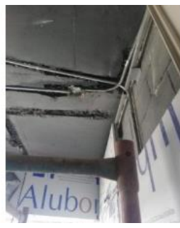
Fig. 15: broken at the ceiling at the skin side Source: Researcher
