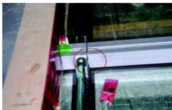
Fig. 4 (B): (Installation issues)Unexpected water ingress at a butt joint in the horizontal mullion during the test chamber Source : [1]
