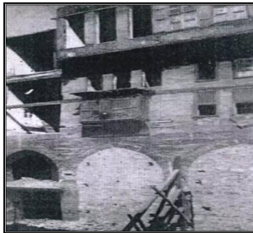
Fig. 19 The condition of the eastern facade overlooking the courtyard deteriorated in 1909
