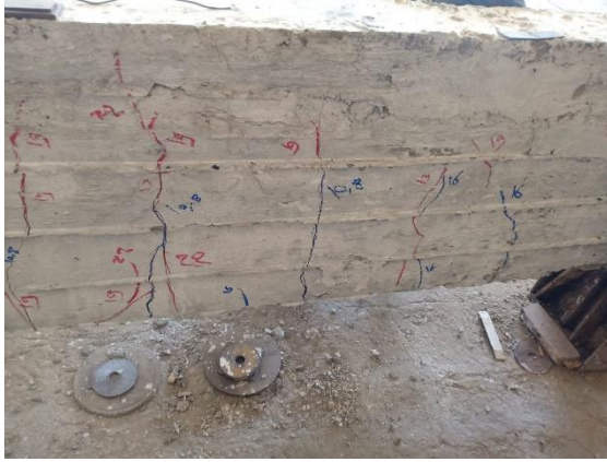
Figure 11 : Crack on the beam (0-350) ( Experimental )
