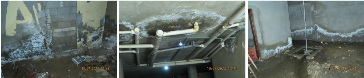
Fig. 12: The problem of ground water in the compound's basements
