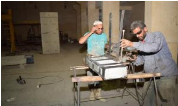
Figure [13] Wrapping the horizontal straps around the column and fixation of straps and angles by welding
