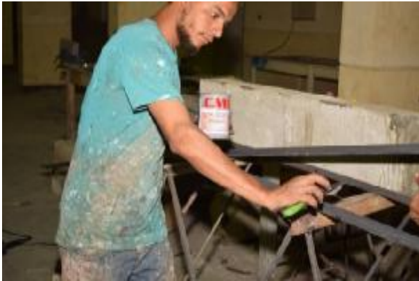
Figure [12] Using epoxy adhesive mortar to ensure full contact between angles and concrete columns
